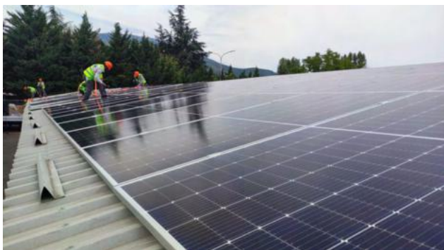
Solar photovoltaic plant at Usje cement plant, North Macedonia.
